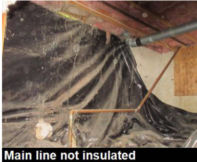
Main line not insulated
