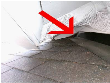
Gap at the house overhang above the garage
