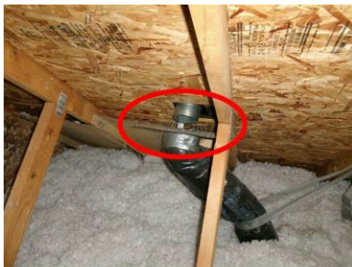
Vent collar unsecured
