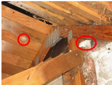
Observed adjacent the chimney in attic
