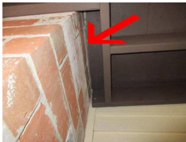
Gap observed adjacent chimney
