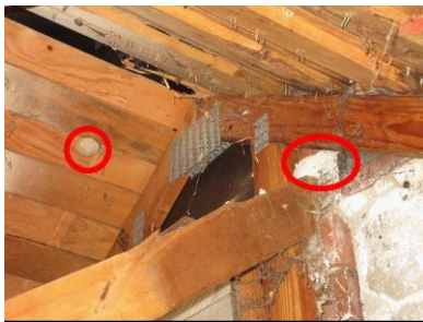
Observed adjacent the chimney in attic
